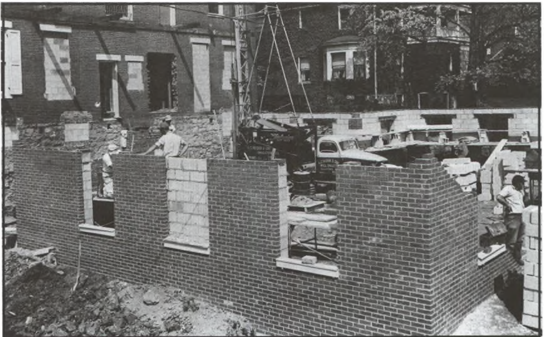
Construction gets under way in 1957 on renovations and an addition to the future Lutheran Home on the West Shore in Camp Hill, Pa.
